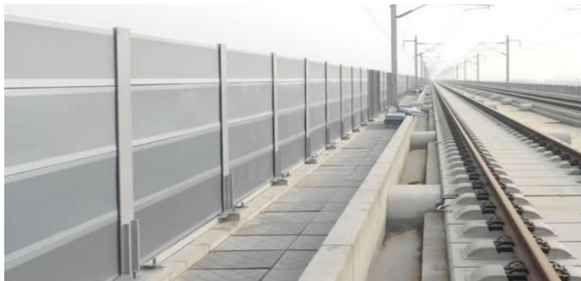
Figure I - 8 Noise barriers should be installed in urban area
