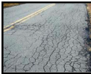
Figure I.2-5 Fissures en carrelage
