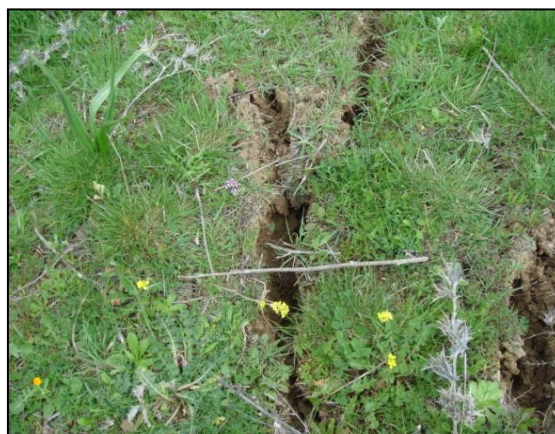
Figure II.4 : Fissuration du talus
