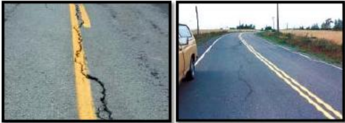
Fig.III.11: fissures de gel
