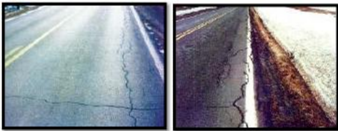
Fig.III.10: fissures de rives
