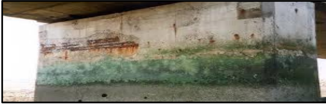
Figure I.1. Carbonatation de béton [1]
