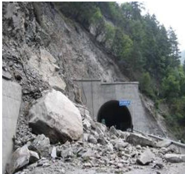
Figure I.10: Classification des dommages sismiques chute des blocs (Shen et al., 2014)
