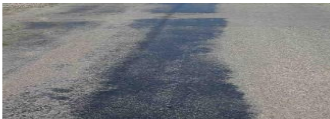
FIGURE 7 RESSUAGE DE LA CHAUSSEE
