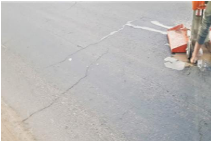
Figure V.20 Fissure transversale au PR 5+500.
