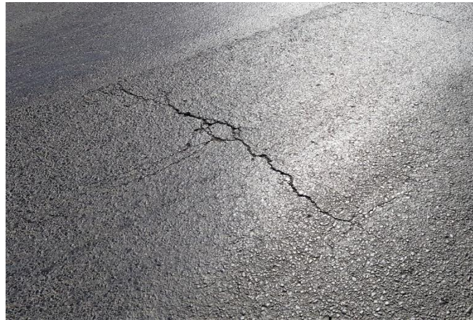
Figure III.23 Les fissures transversales.
