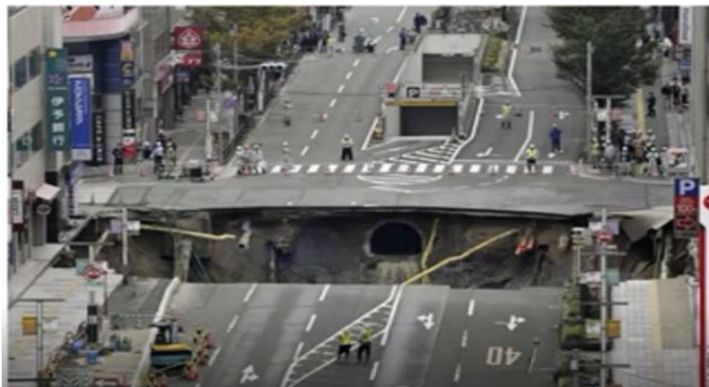
Figure II.4 Exemple de rupture (effondrement) [S18]
