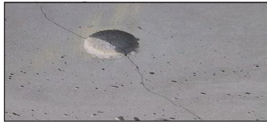
Figure I.10 Fissuration du béton
