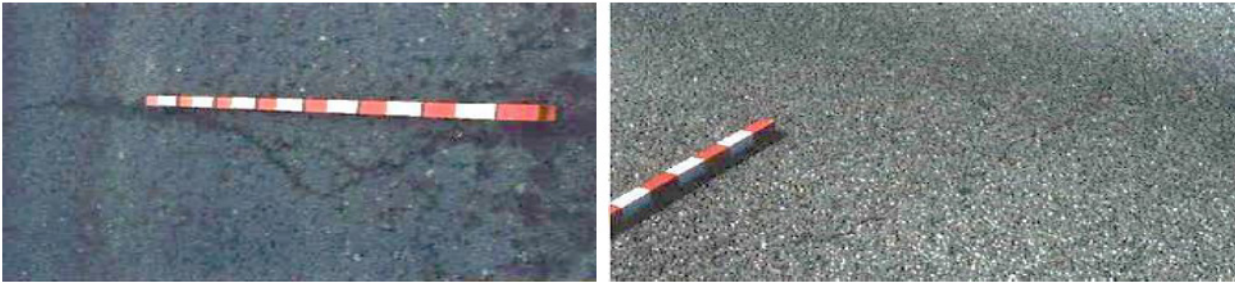
Figure 11: Exemples de fissuration transversale
