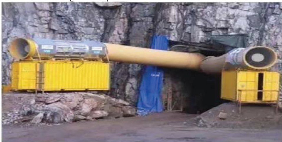
Figure I-17 : turbine de ventilation
